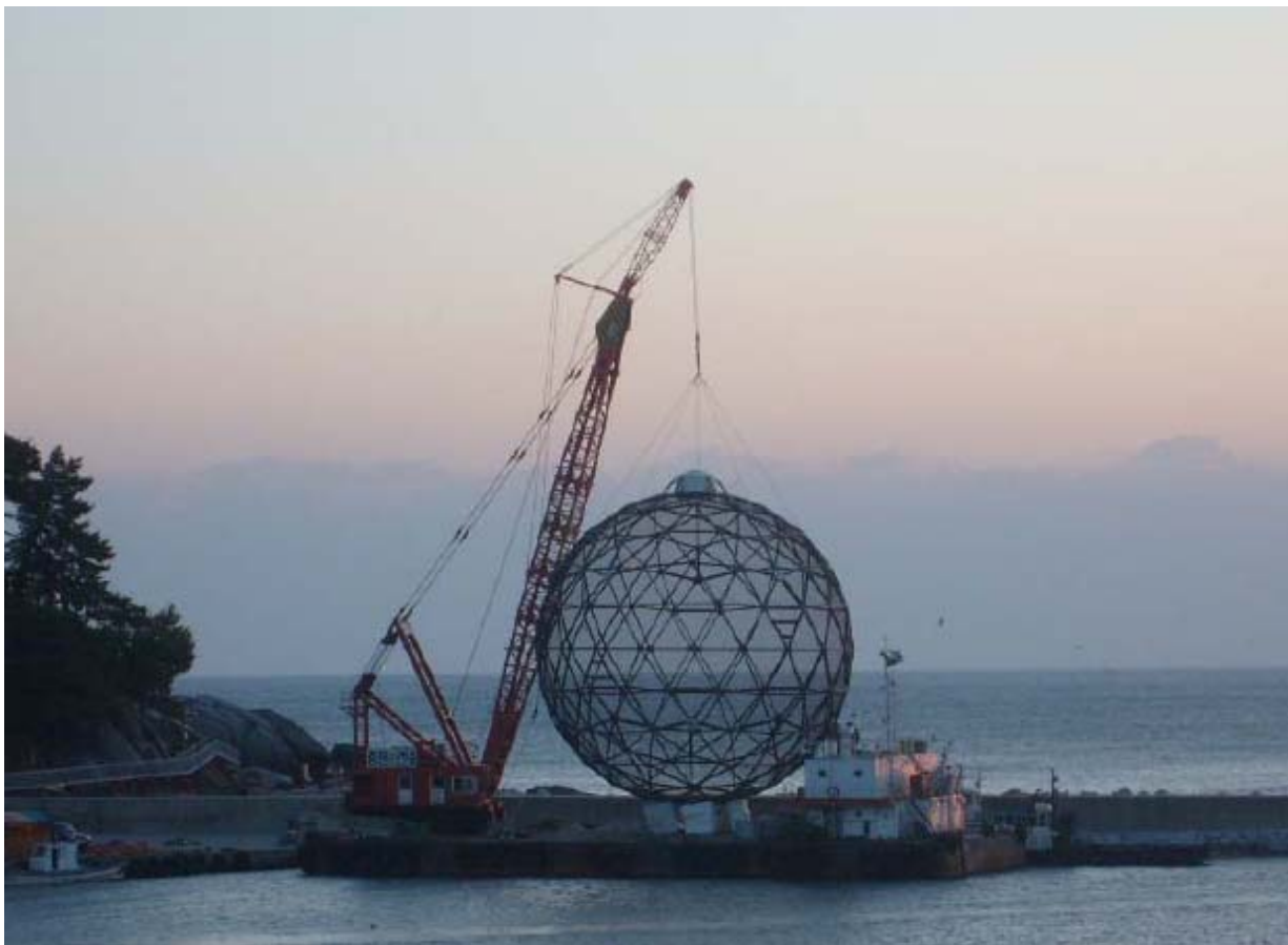
An A3600 Aquapod positioned on a crane barge at sunrise in Yangyang, South Korea.
